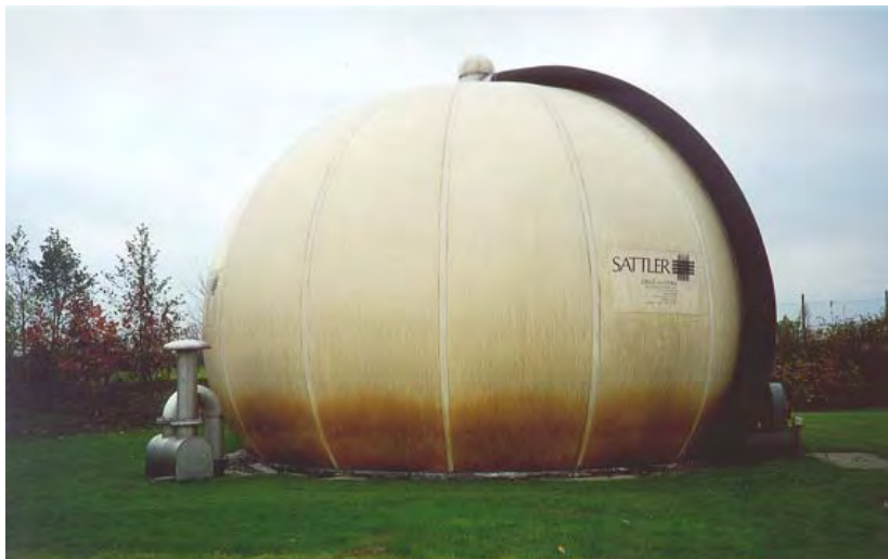
Plate 5.5 Anaerobic Digestion Plant
